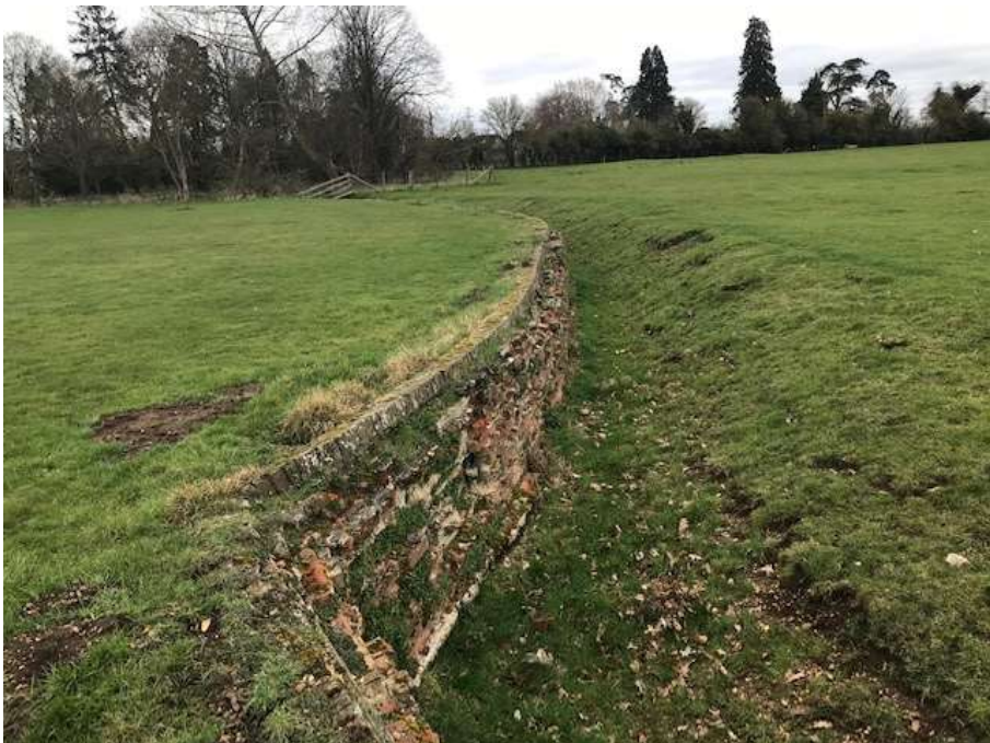
Image 2: Looking south along the post-medieval ha-ha (MBB22347) within former parkland (MBD9067) in the Site, west of Barford Road
