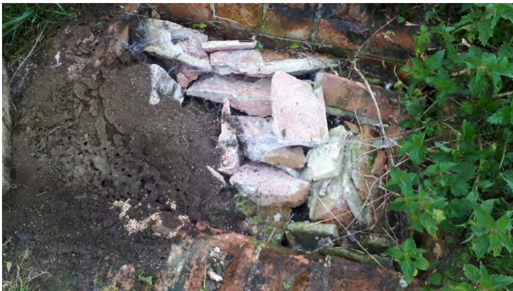
Photo 12. Abandoned drainage chamber filled in with rubble, located to south of farmyard (see Figure 2 for location).
