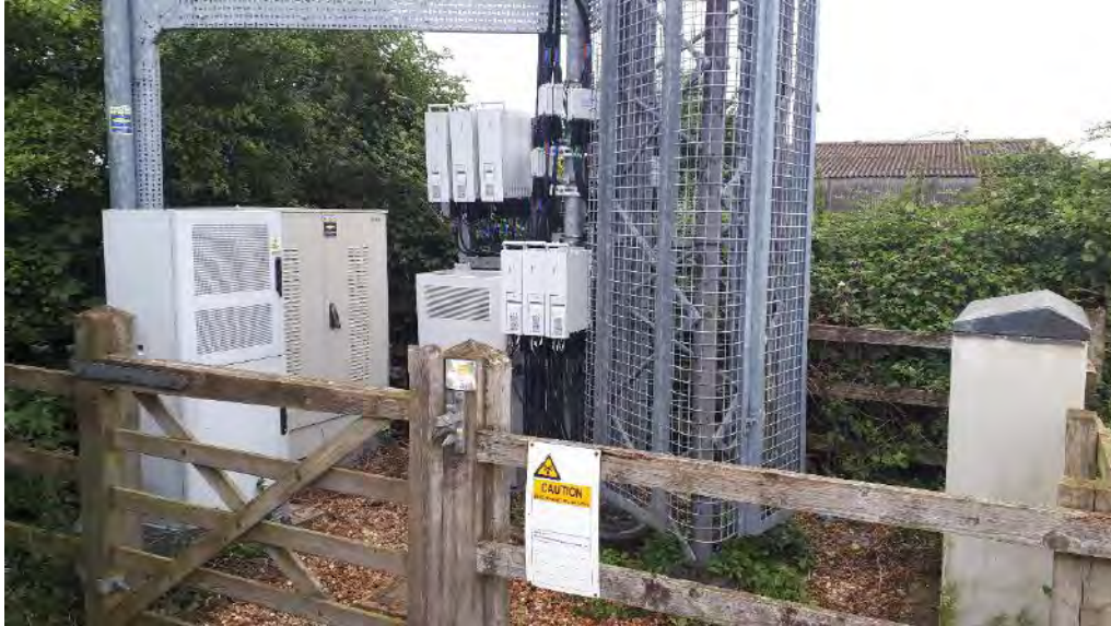
Photo 7. Telecommunications mast in west of farmyard (see Figure 2 for location).
