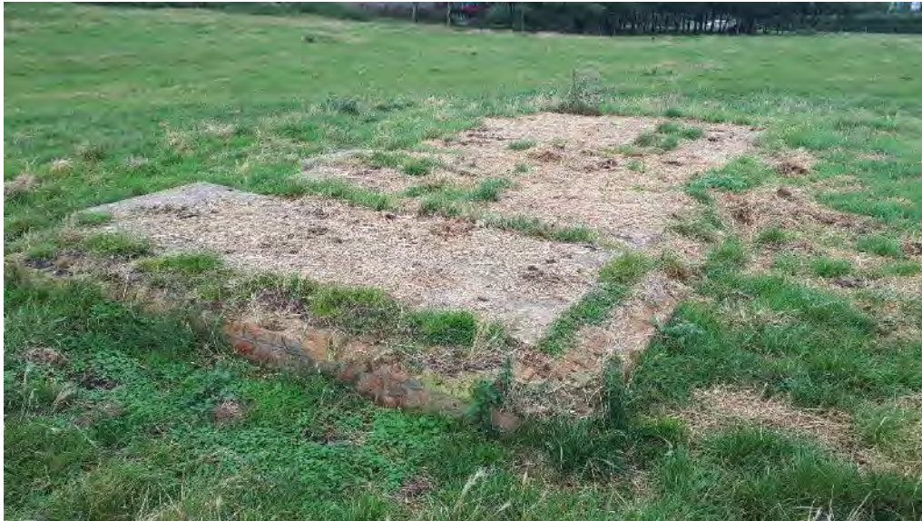
Photo 11. Abandoned foundation of 'shower block' located to south of farmyard (see Figure 2 for location).
