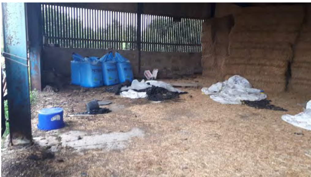
Photo 4. Building 3, photo facing east. Steel A frame shed with corrugated cement cladding, used as cattle pen and fertiliser storage (blue bags) (see Figure 2 for location).
