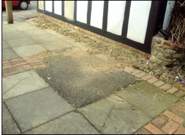
Figure 36. Unsympathetic repairs to paving on Bunyan's Mead
