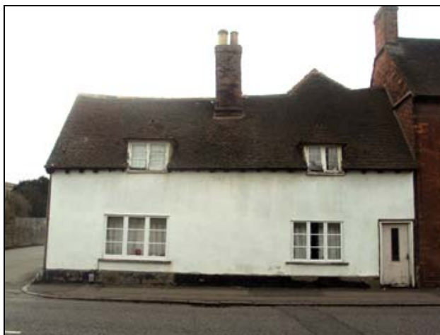
Figure 34. Green Corner, a property in need of some maintenance
