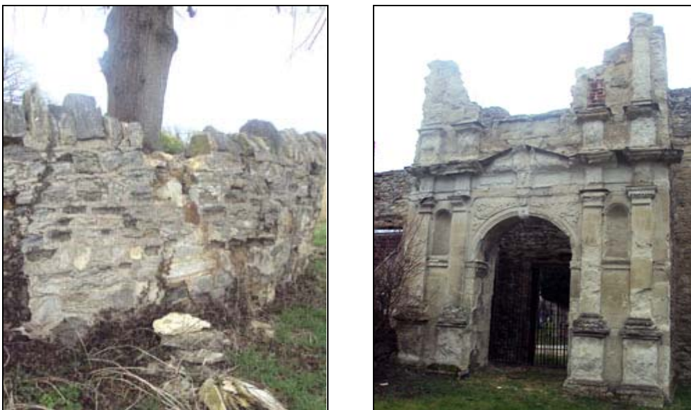
Figure 47. Damage to churchyard boundary wall (left) The Renaissance porch to Elstow Place - in an 'at risk' condition (right)
