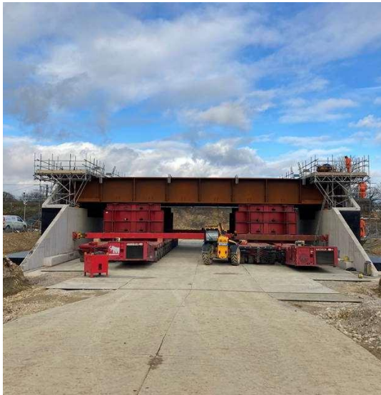
Figure 3.2: NW Bicester Off line abutments and rail deck ready to be installed
