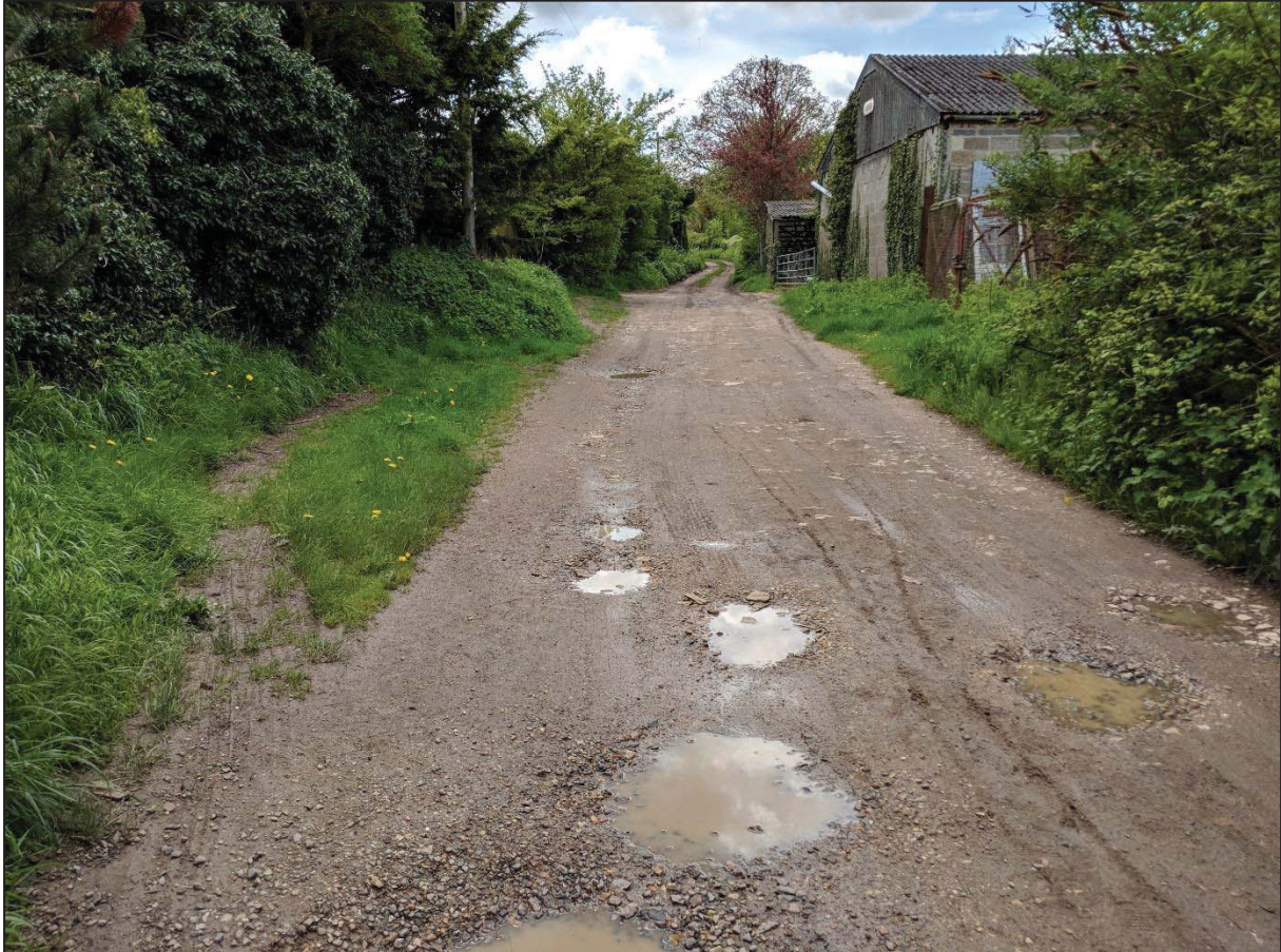
Figure 2: Town Lot Lane Surface Conditions
